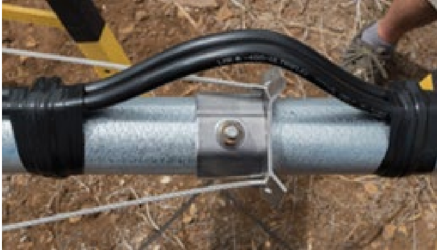
Figure 9—Coaxial cable fed around guy bracket
